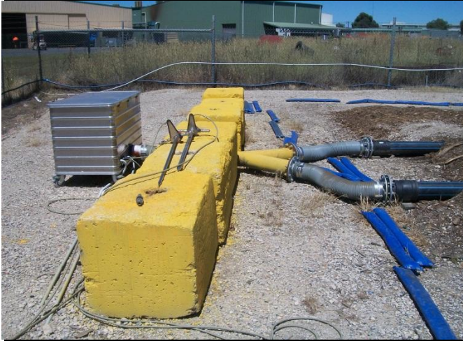
Aeration equipment, manifold and probes
