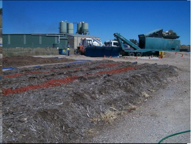
Organic bed with woody material containing the aeration pipes
