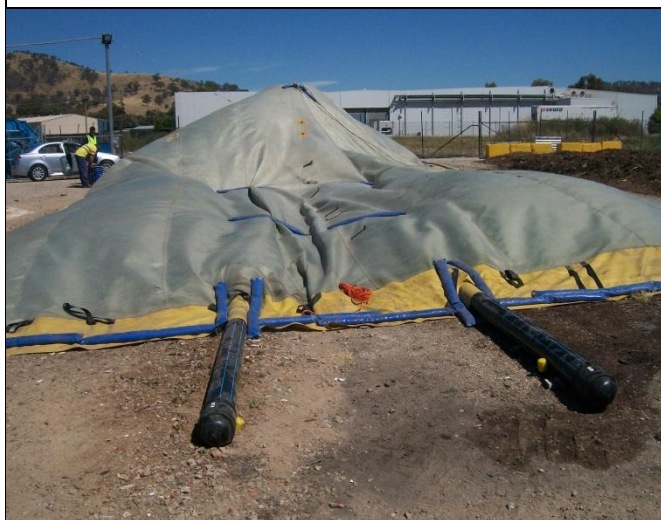
Aeration pipes in base of windrow
