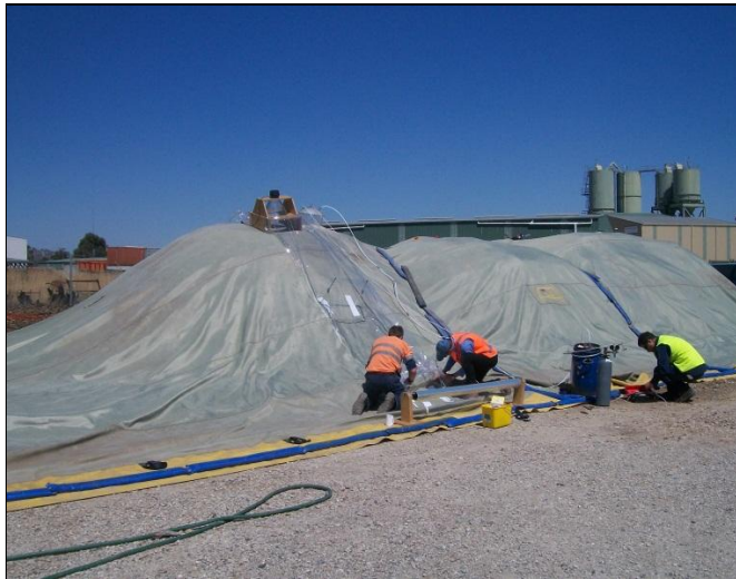
Installation of air sampling equipment
